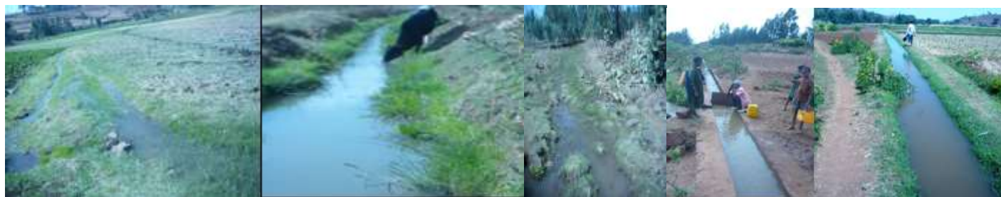
Figure 2. Overflowing of unlined canals and livestock interference at Selamko (left 3) and lined and unlined main canals at Shina-Hamusit (right 2) irrigation schemes.
